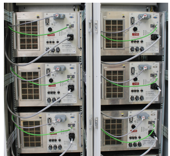
Cabinet with Switch Mode Power Supplies
